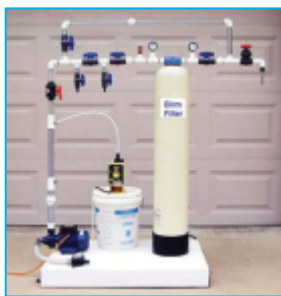
Iron Removal System (Birm Filter)
