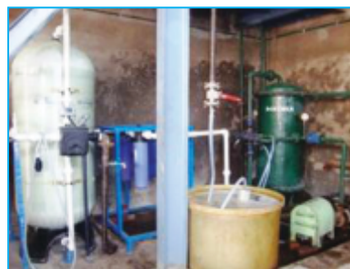
Soft Water Plant (Auto / Manual)
